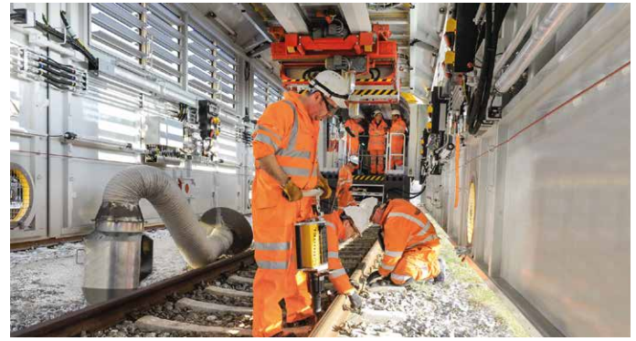
Fig. 4: An overhead crane, ventilation, lighting and the use of hand-operated battery-powered machines provide for maximum ergonomics and work safety in the mobile maintenance system.
