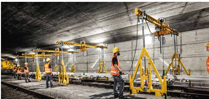
Fig. 1: Replacement of switches/rails in tunnels without a crane: Automatic positioning system for the London Elizabeth Line.
