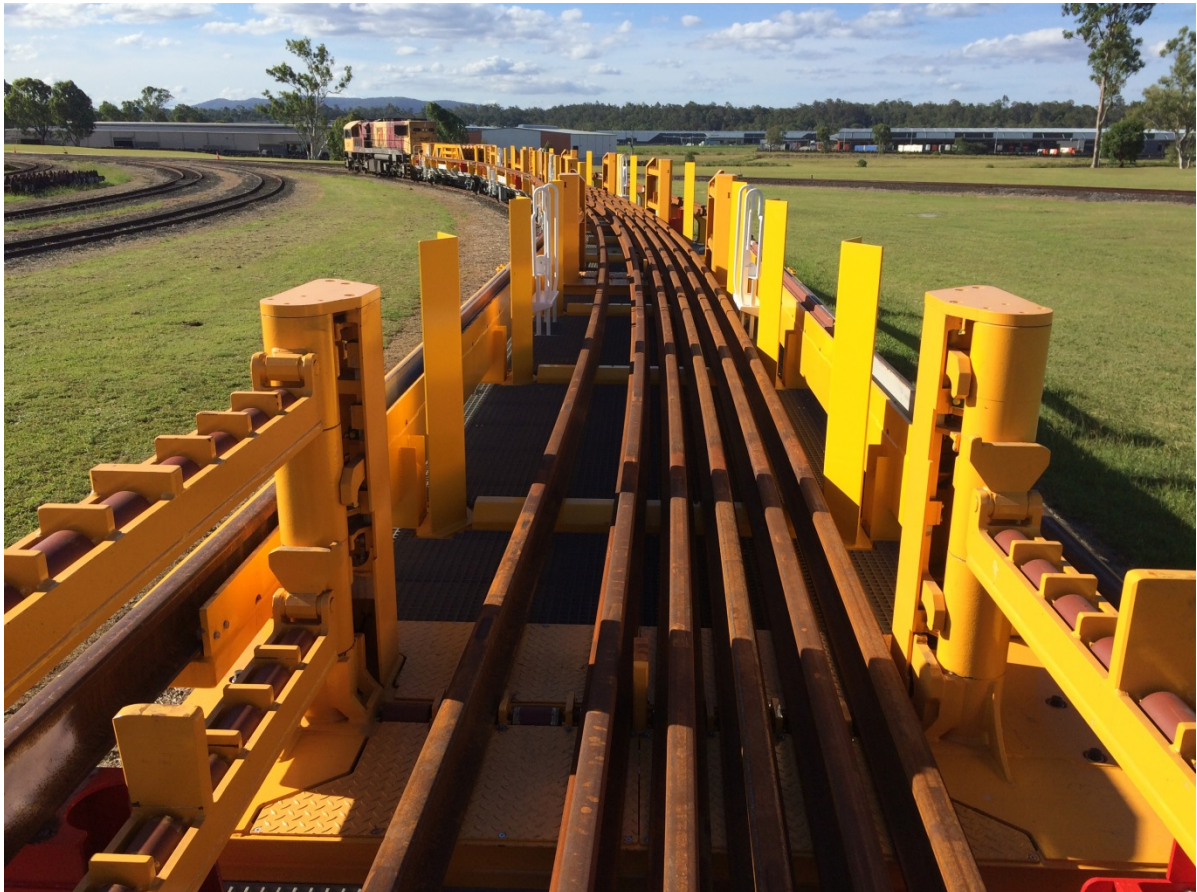
Fig. 9: Up to 50 rails with a maximum length of 500 m are transported safely, adhering to the bending limits and yield points.
