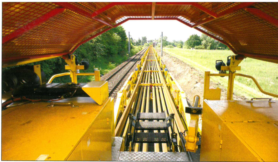
Above: Rear view from the manipulator showing the long welded rail strings on the train's wagons.
