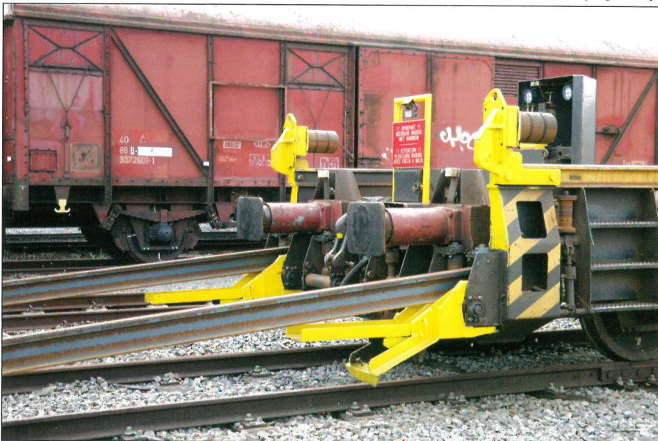
Below: Rail delivery from the end wagon of the train showing the resilience chutes (in yellow).
